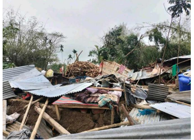
picture 1: The destruction after the Nor'wester storm hit Haluaghat, Mymensingh
